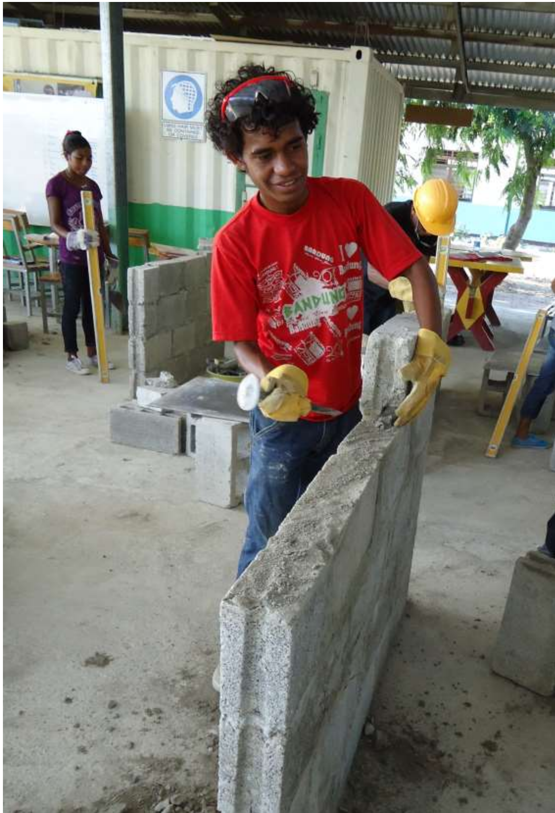
Building Construction students at Don Bosco Technical Training Centre, Comoro, Timor Leste.
